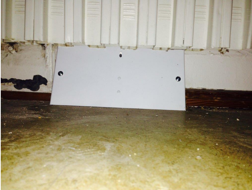
Tilluftsdon under radiator.
