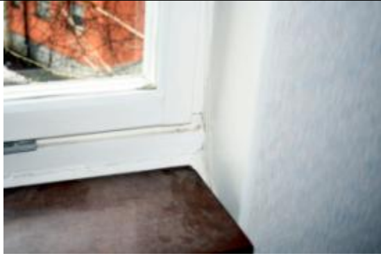
Figure 5a. Leak through window frame.
