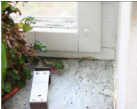
Figure 6a. Leak trough window frame and arch.
