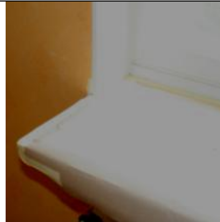
Figure 4b. Leak through window frame and arch.
