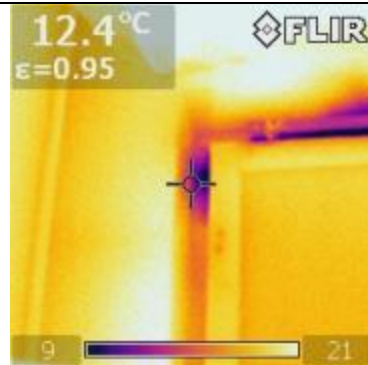
Figure 4b. Leak between window frame and arch.
