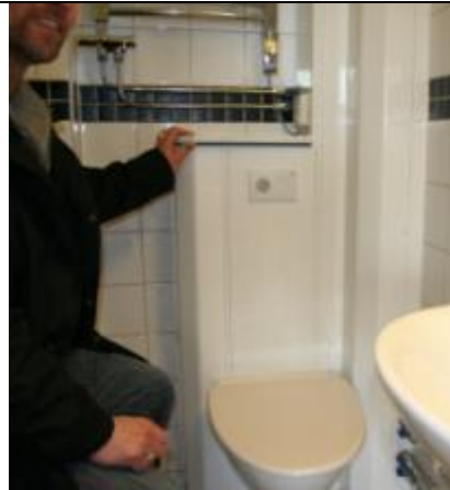
Figure 7a. An air leakage was measured with hot wire anemometer through opening of cover to the WC shaft. 0.3 m/s was indicated.
