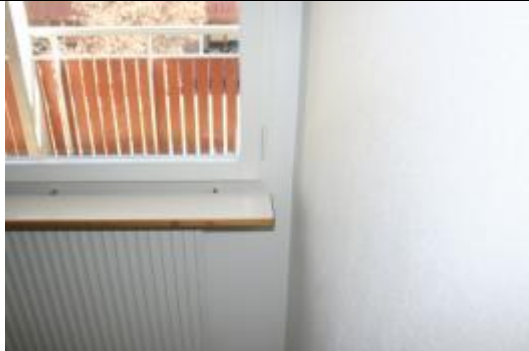
Figure 14a. Kitchen. Leak between window frame and arch.
