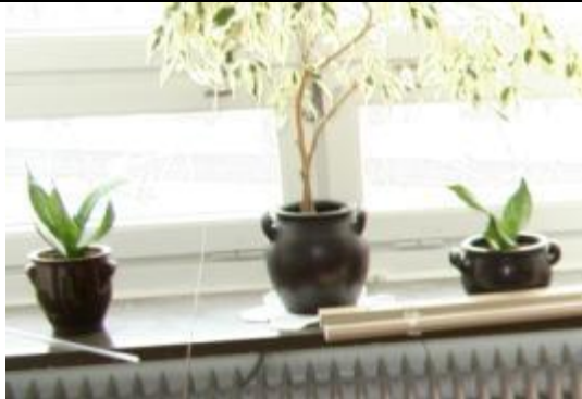
Figure 6a. Bed room, leak trough window frame and arch.
