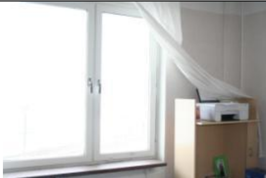
Figure 2a. Leak between windowframe and arch.
