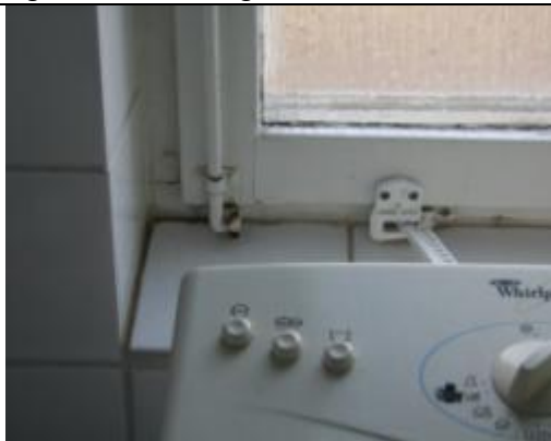
Figure 7a. Leak trough window frame and arch.
