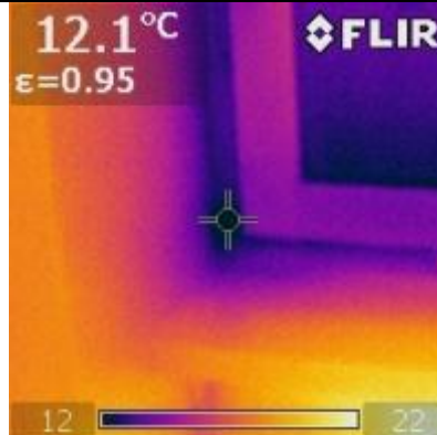
Figure 8a. Leak between window frame and arch.
