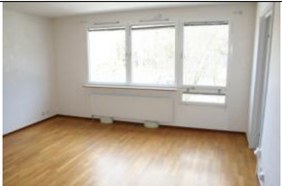
Figure 9a. Original balanced mechanical ventilation with supply air devices ("Elephant foot") in floor have been changed with exhaust air ventilation with exterior air devices (Biobe) in window frame. The old supply air system is not sealed and it is possible for air change between apartments. The measurements showed an air change between apartments of about 33 l/s, ( 9+9+15=33 l/s).
