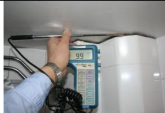
Figure 10b. In crack to ducts was air speeds measured around 1m/s that probably depend on leaking air from the neighbor. Under pressure in the apartment was constant at -50 Pa during this measurement. (Water pipes were changed in 2005)
