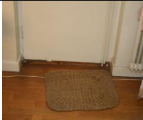
Figure 2a. Leak at balcony door.
