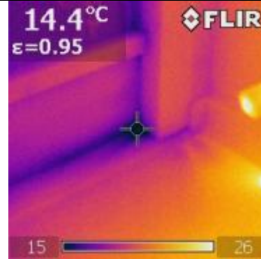
Figure 6b. Leak between window and floor.
