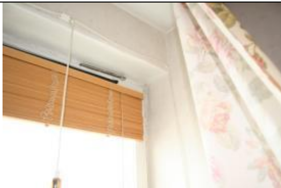
Figure 3a. Bed room, leak trough window frame and arch.
