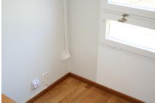
Figure 5a. . Living room, leak in corner between skirting-board and floor.
