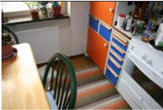
Figure 4a. Kitchen, leak between skirting-board and floor.
