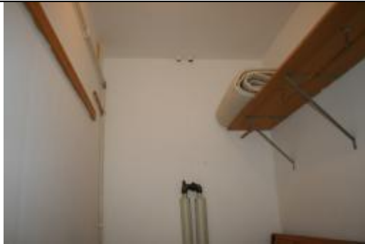
Figure 6a. Two cut offed pipes in the ceiling in cloths cupboard.
