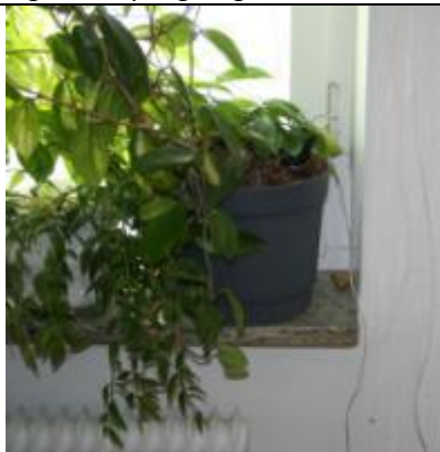
Figure 2a. Leak trough window frame and arch.
