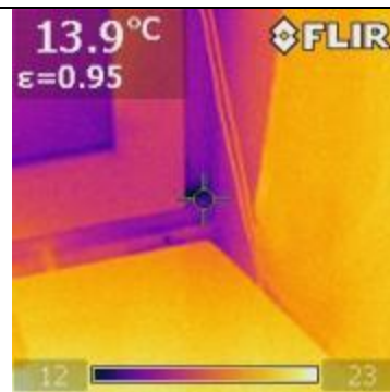
Figure 2b. Living room, leak trough window frame and arch.
