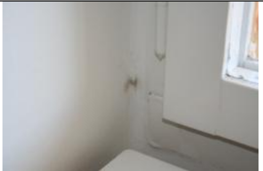
Figure 15a. Kitchen. Leak between window frame and arch.
