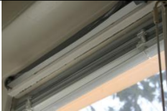
Figure 4a. Leak between external air device and window arch.
