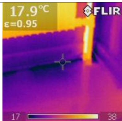
Figure 7a. Leak between skirting-board and floor.
