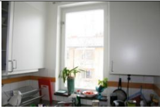
Figure 4a. Kitchen, leak trough window frame and arch.
