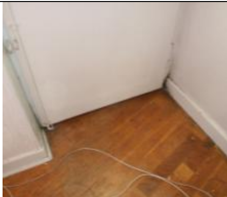
Figure 3a. Leak through balcony door (between arch and frame/ doorstep).
