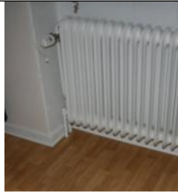
Figure 5b. Bed room, leak between skirting-board and floor.
