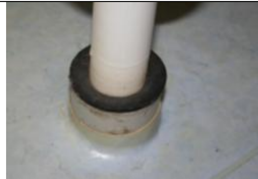
Figure 16b. Bath room. Leak through sewage pipe from washbasin and sewage pipe in joists. This is probably the reason for sewage smell in the bath room since water seal was full with water.
