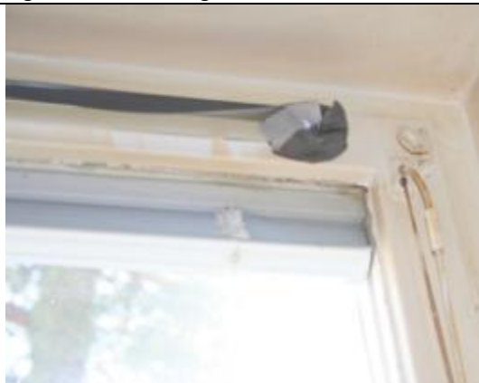
Figure 4a. Leak trough window glas and arch and between frame and arch.
