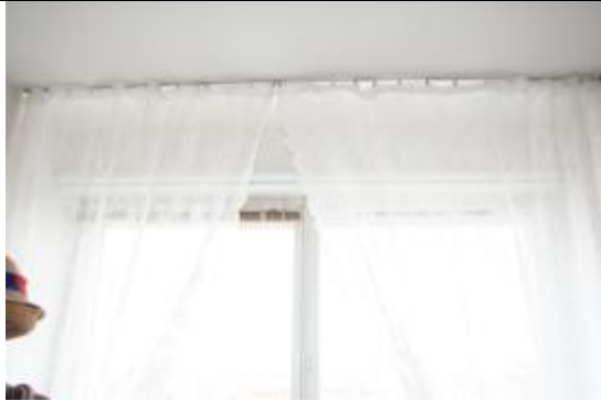
Figure 5a. Bed room, leak trough window frame and arch.
