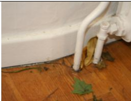
Figure 4a. Leak between skirting-board and floor.
