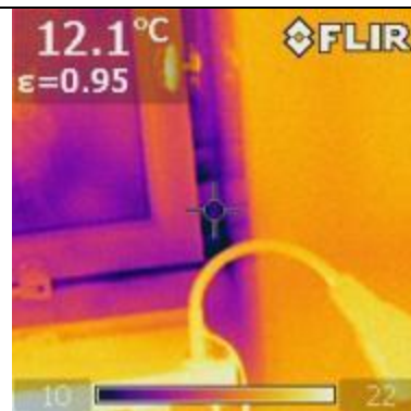
Figure 5. Leak trough window frame and arch.
