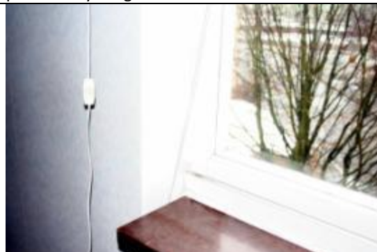
Figure 4a. Leak trough window frame and arch.
