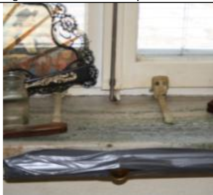
Figure 3a. Leak trough window frame and arch.
