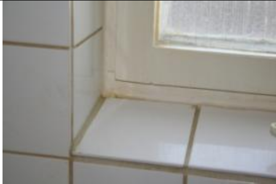
Figure 6a. Leak trough window frame and arch.
