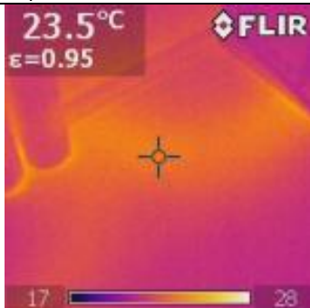
Figure 19a. Even though supply water temperatures is relatively low could surface temperatures of floor be measured to 23,5°C, due to heat losses from water pipes.
