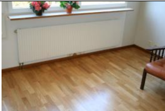
Figure 2a. Living room. Installation of new floor hides two supply air openings from an old supply air system. Now its renovated to anexhhaust air system.
