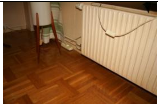
Figure 2b. Living room. Leakage was registered through splice between external wall and floor.
