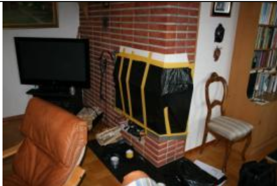
Figure 7. Air tightness testing were performed both with sealed stove and unsealed stove. No measurable difference in air flows were registered. The smoke damper, which was closed in both measurements, is obviously air tight.
