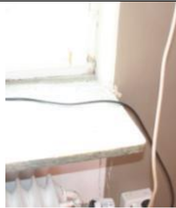
Figure 3b. Leak through window frame and arch.
