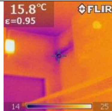
Figure 8b. Leak throgth bushing for electrical cable.
