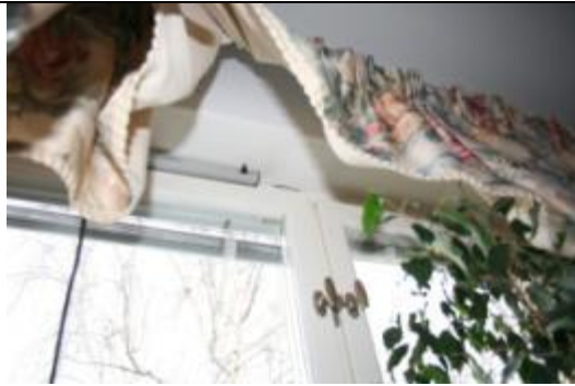
Figure 10a. Leak trough window frame and arch.
