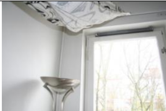
Figure 4a. Leak between window frame and arch.
