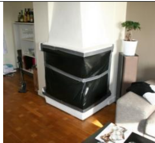
Figure 5b. No measurable difference in air flows were registered between sealed and unsealed stove.
