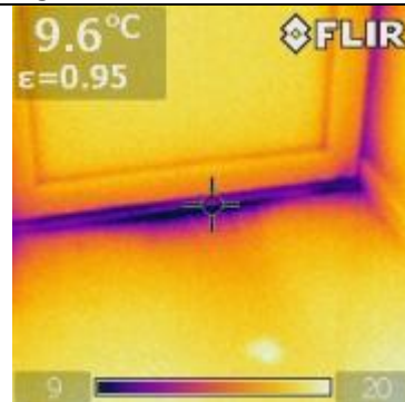
Figure 7b. Balcony door, leak between doorstep and floor.
