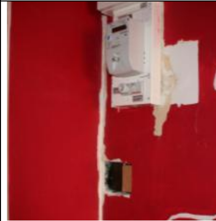
Figure 7b. A smaller air leakage was indicated within the electrical control unit.
