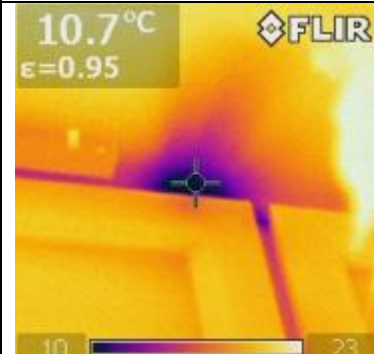
Figure 10b. Leak trough window frame and arch.
