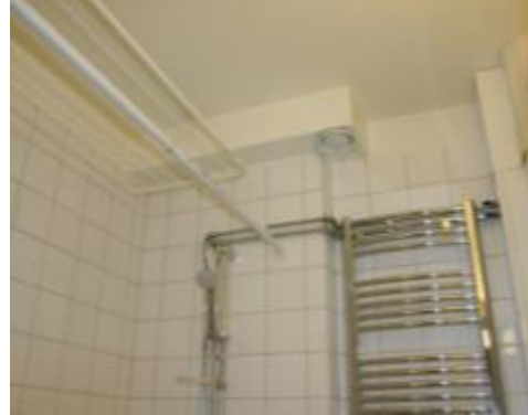
Figure 8b. Exhaust air device in bath room and horizontal duct to exhaust air device in living room.
