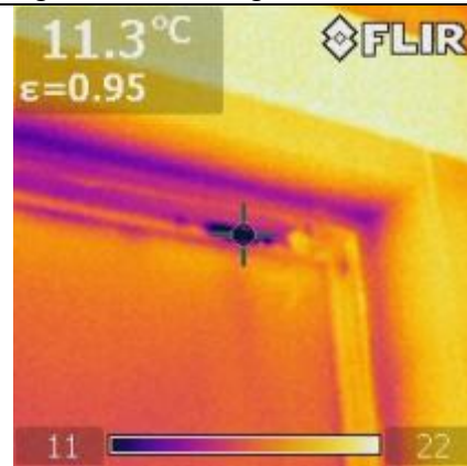
Figure 4b. Leak trough window glas and arch and between frame and arch.
