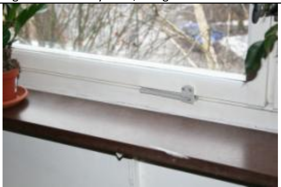
Figure 8a. Leak trough crack in window frame.
