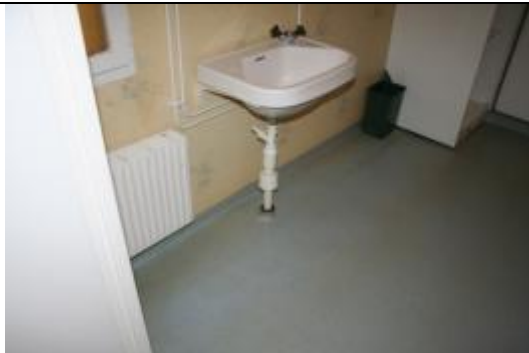
Figure 16a. Bath room. Leak through sewage pipe from washbasin and sewage pipe in joists. This is probably the reason for sewage smell in the bath room since water seal was full with water.
