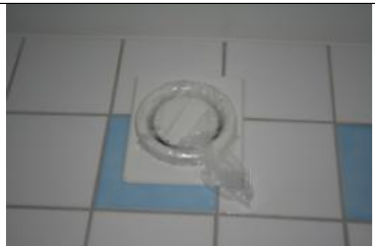
Figure 2b. At air tightness tests were external air devices and exhaust air devices temporarily tightened.
