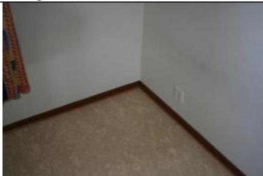
Figure 10a. Bed room, leak in corner between skirting-board and floor.
