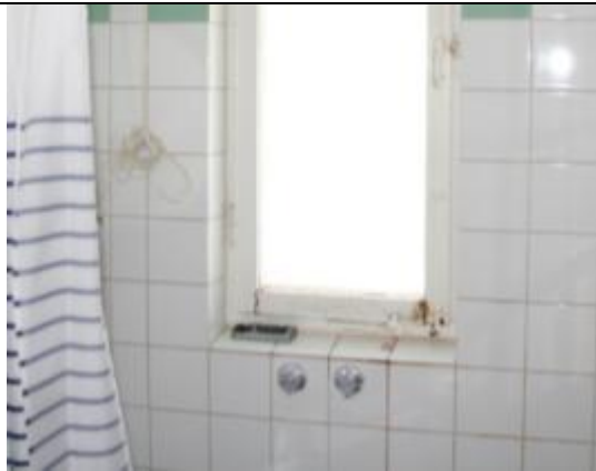
Figure 3a. Bath room, leak trough window frame and arch.
