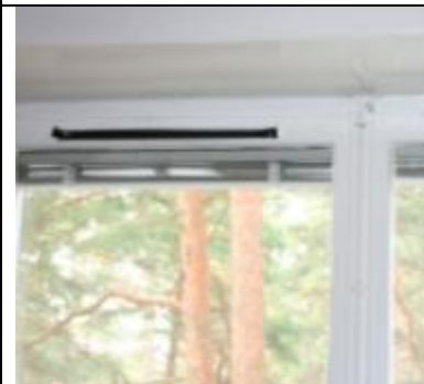
Figure 2b. Leak through crack between external air device and window arch.
