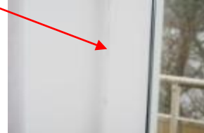
Figure 6c. Crack in door frame.
