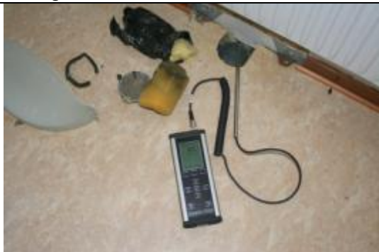
Figure 11a. Supply air device in bed room was temporary sealed with glass wool and foam plastic. Without sealing was an air speed of 4 m/s measured in the opening and an air temperature of +20°C, which indicates that it is air from neighbor apartment.
