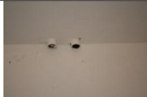
Figure 6b. Two cut offed pipes in the ceiling in cloths cupboard.
