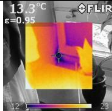
Figure 6b. Bed room, leak trough window frame and arch.
