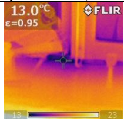
Figure 3a. Leak trough window frame and arch.
