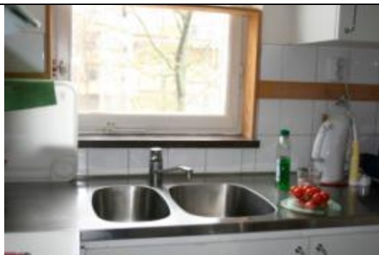
Figure 8a. Kitchen, leak trough window frame and arch.
