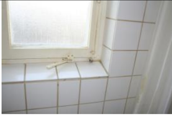
Figure 5a. Leak trough window frame and arch.
