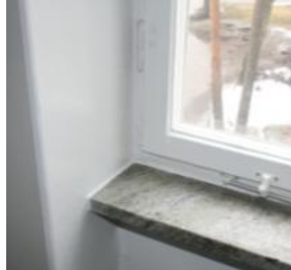
Figure 8b. Leak between window frame and arch.
