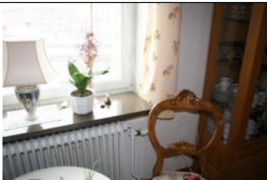
Figure 2a. Living room, leak trough window frame and arch.
