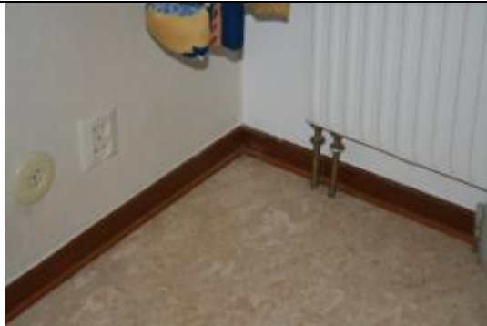
Figure 9a. Bed room, leak in corner between skirting-board and floor.
