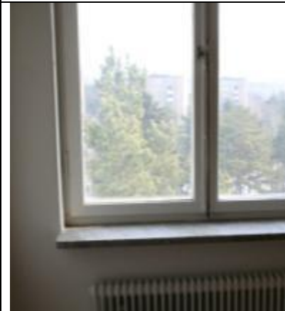
Figure 6b. Leak through window frame and between frame and arch.
