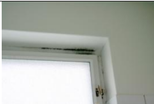
Figure 2a. Bed room, leak trough window frame and arch.
