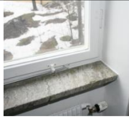
Figure 9b. Leak between window frame and arch.
