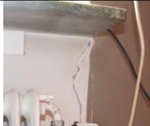
Figure 2b. Leak through crack in exterior wall.
