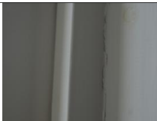
Figure 9a. Living room. Crack between window frame and external wall.
