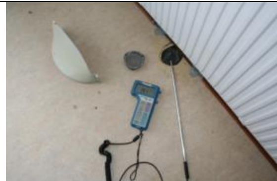
Figure 9b. In bed room was air speeds of 2 m/s measured in supply air opening (air from the other apartment). 2 m/s correspond to about 9 l/s in the opening.
