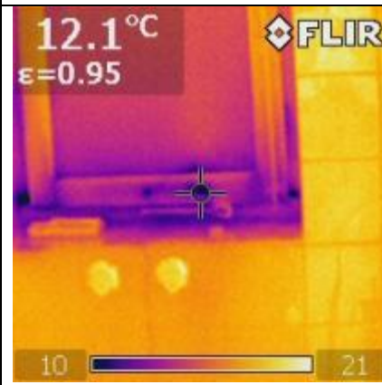
Figure 3b. Bath room, leak trough window frame and arch.
