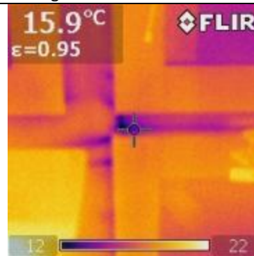
Figure 3b. Leak between window frame and arch.
