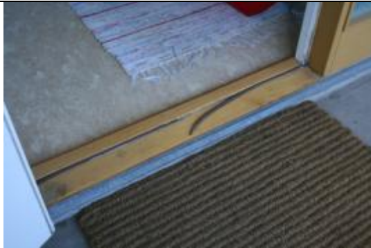
Figure 17. Front door. Leak through broken weather strip.
