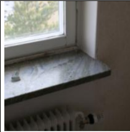
Figure 5b. Leak through window frame and arch.
