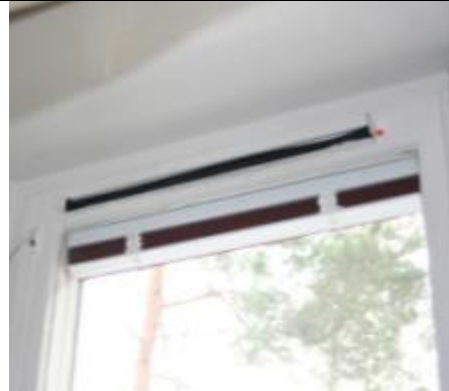
Figure 6b. Leak between external air device and window arch.
