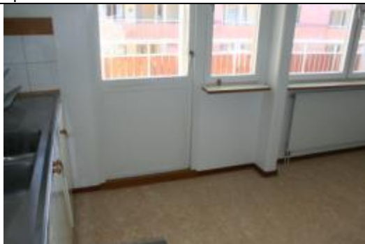
Figure 12a. Kitchen. Large leak between balcony door and door frame.
